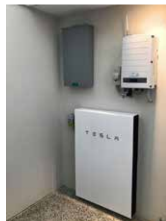
Tesla home storage battery
