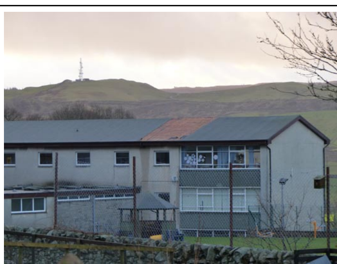
Above is a photograph of the damage to Dalry school roof caused by storm Eleanor on the night of 2-3 January, submitted by Paul Goodwin.
